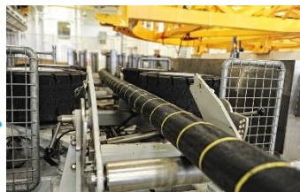
Hornsea One Windfarm (UK)
